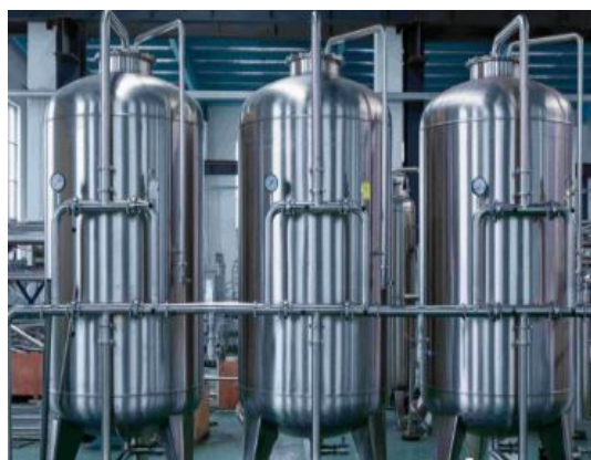
Pic.1 Water filter system
